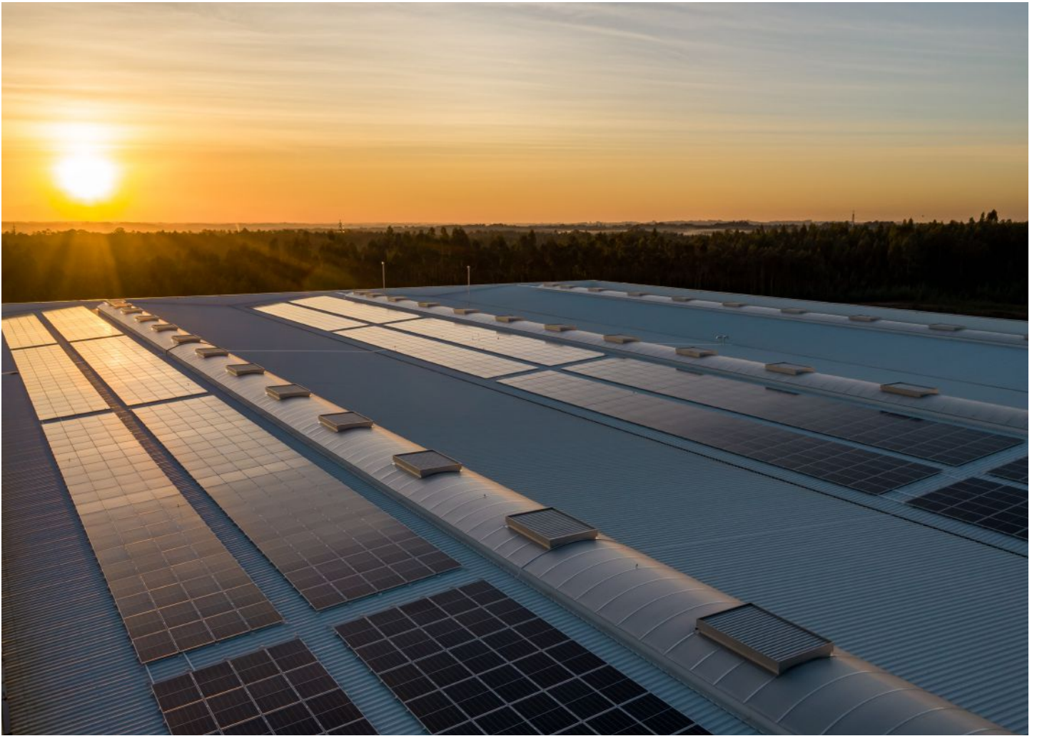
Manufacturing facility with rooftop solar installation
